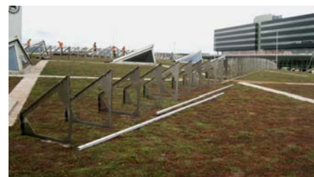
The Solar Base Frames were well adapted to the slight inclination of the roof construction.
